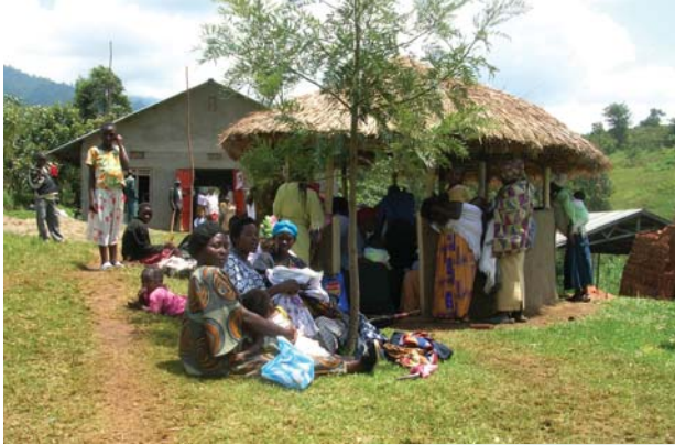
Maternity ward under construction, at the Rambia Health Centre, near Fort Portal.
